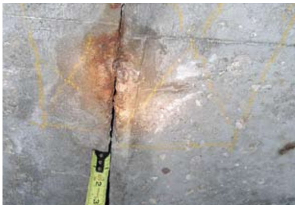
Fig. 2: Differential in the elevation of the bottom of the slab at the construction joint
